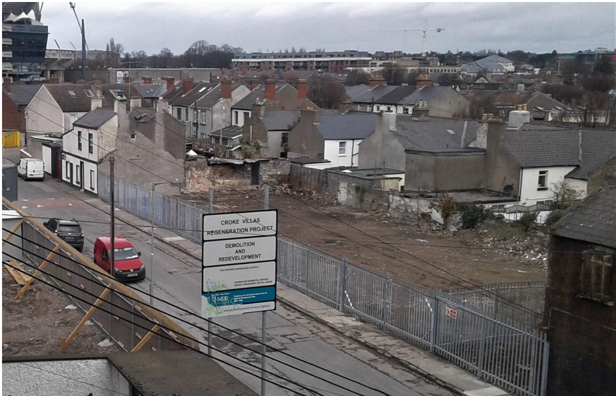
Demolition work on the former cottages on Sackville Avenue is now completed and the two sites cleared.
